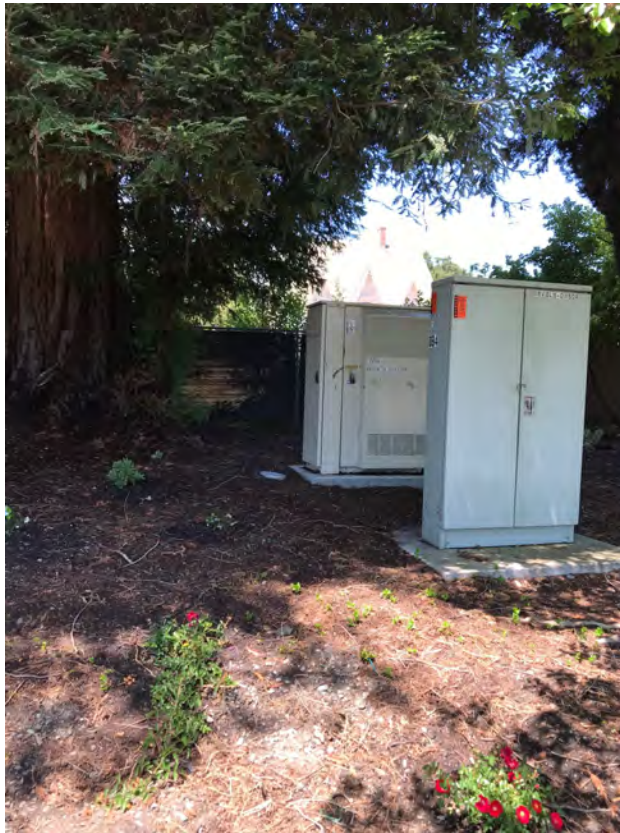
Photo 26 – Two utility vaults, San Ramon Valley Blvd, adjacent to east fence
