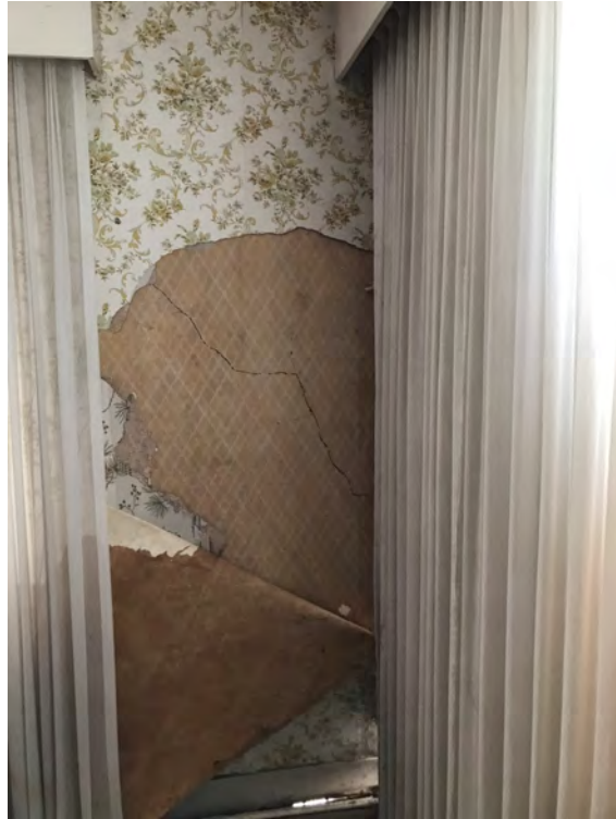
Photo 3 – House, peeled wallpaper, cracked wall board, east wall 1st floor l
