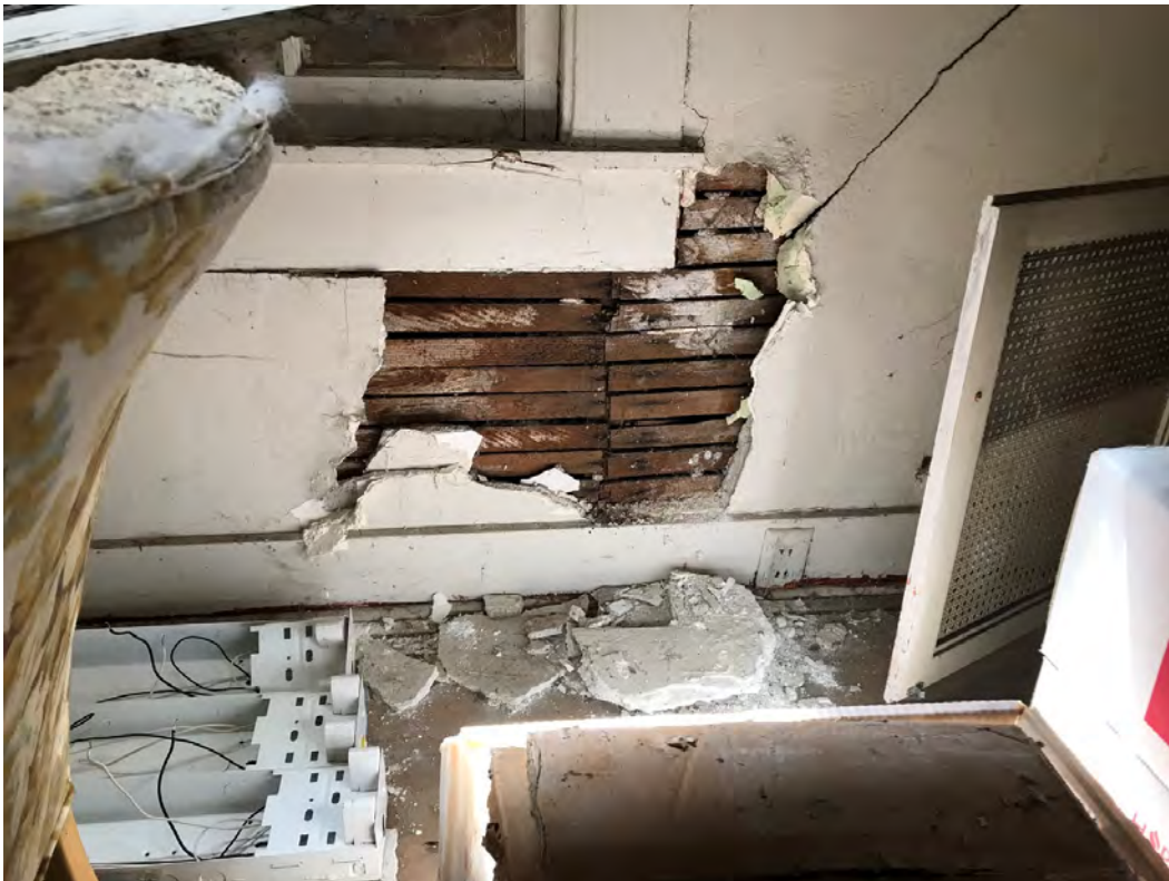
Photo 4 – House, broken drywall, south wall, 1st floor by staircase
