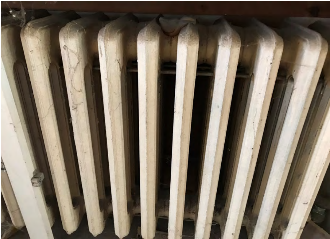
Photo 2 – House, radiant heater, east wall 1st floor
