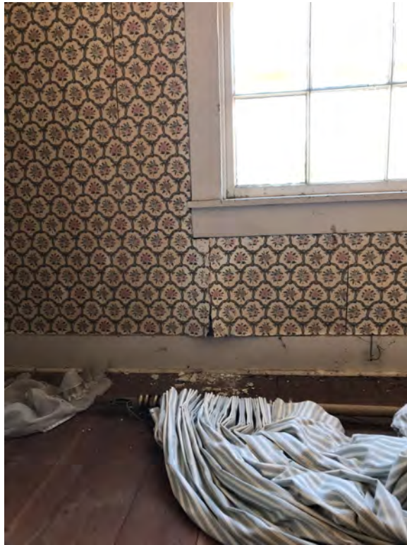
Photo 5 – House, North wall, 2nd floor, broken drywall
